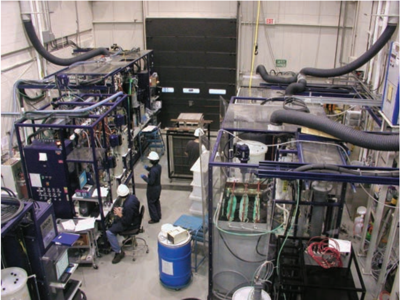
Figure 7: POL Process Miniplant at Mississauga, Ontario (Courtesy of Vale).
